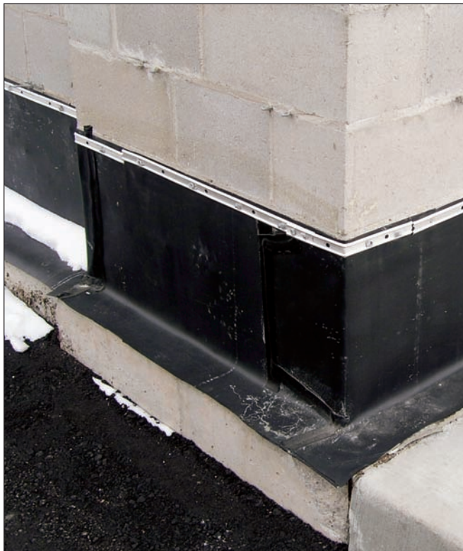
The above photo illustrates a flush-applied ethylene propylene diene monomer (EPDM) installation with termination bar and sealed laps. (Note: the sealant atop the termination bar has yet to be installed.)
